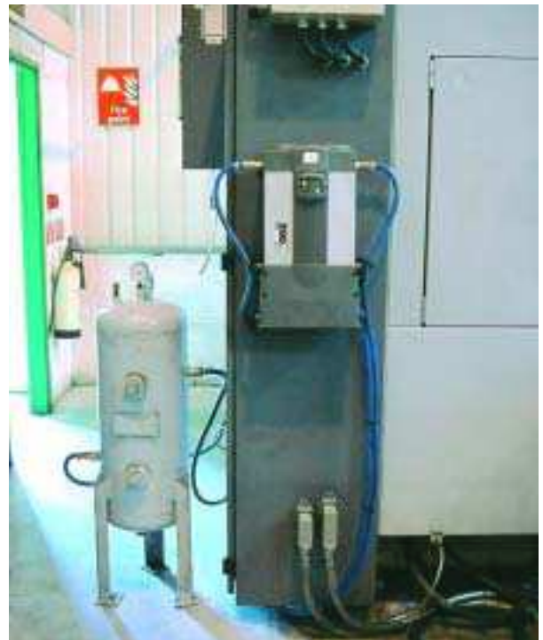
PNEUDRI MiDAS installed to supply control air for a CNC machining centre
