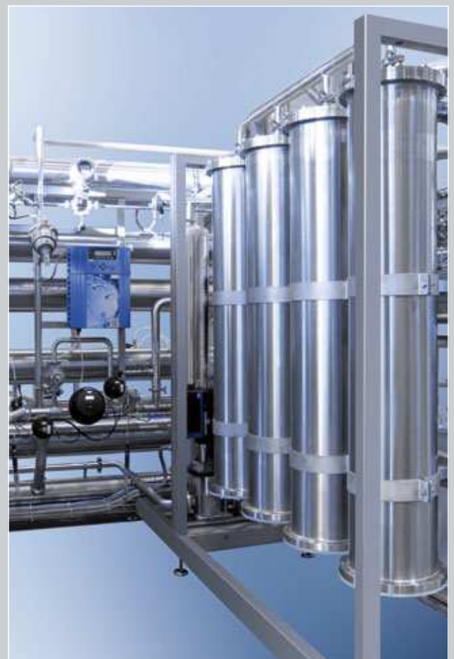
All aggregates and components are perfectly accessible for maintenance work.
