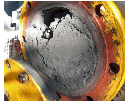
Black Powder accumulated in gas transmission pipeline. Image courtesy of ROSEN Group
